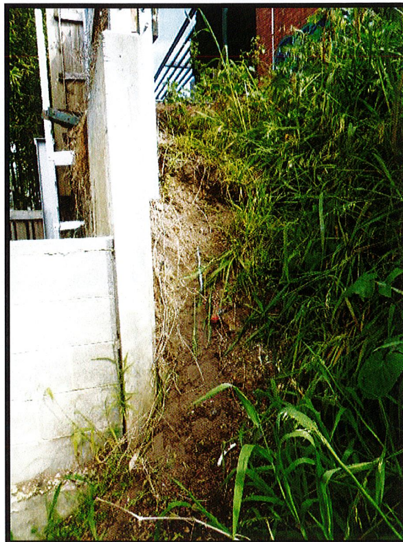
Photograph 10 – Photograph captured 13 October 2021. View of the western end of the subject land, looking west, at the north-east corner of 1 Campbell Grove (north-east corner of 1A Campbell Grove). Erosion of ground adjacent to retaining wall evident compared to November 2020 (photographs 7 – 9).
