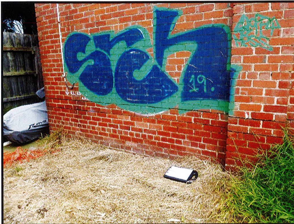
Photograph 20 – Photograph captured 13 October 2021. No evidence of movement and / or damage to the brickwork wall along the south boundary of 42 James Street, at the top of the battered ground to the subject land.
