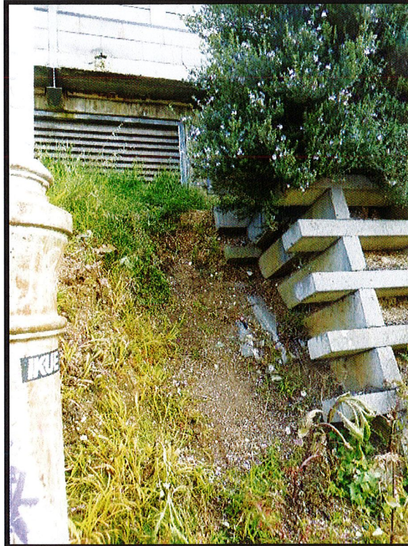
Photograph 6 – Photograph captured 14 October 2021. View of the eastern end of the subject land, looking north. Note localised erosion of land resulting in steep slope adjacent to crib wall.
