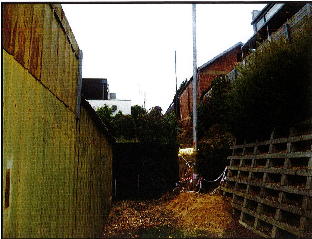
Photograph 2 – Photograph captured 29 April 2019. View of eastern end of subject land, looking west. Note spoil / loose material in laneway at the bottom of the batter.
