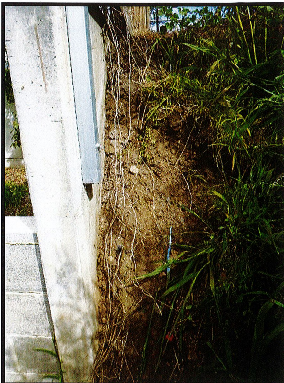
Photograph 11 – Photograph captured 13 October 2021. View of the western end of the subject land, looking west, at the north-east corner of 1 Campbell Grove (north-east corner of 1A Campbell Grove). Erosion of ground adjacent to retaining wall evident compared to November 2020 (photographs 7 – 9).
