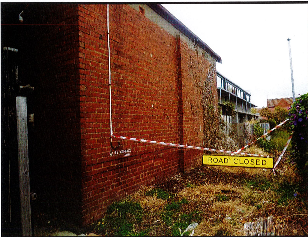
Photograph 18 – Photograph captured 29 April 2019. No evidence of movement and / or damage to the brickwork wall along the south boundary of 42 James Street, at the top of the battered ground to the subject land.
