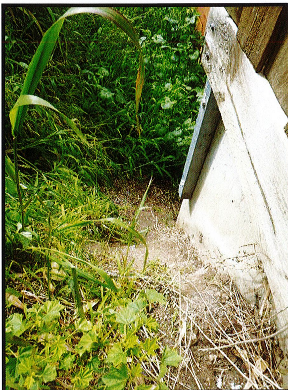
Photograph 12 – Photograph captured 13 October 2021. View of the western end of the subject land, looking east, at the north-east corner of 1 Campbell Grove (north-east corner of 1A Campbell Grove). Erosion of ground adjacent to retaining wall evident compared to November 2020 (photographs 7 – 9).
