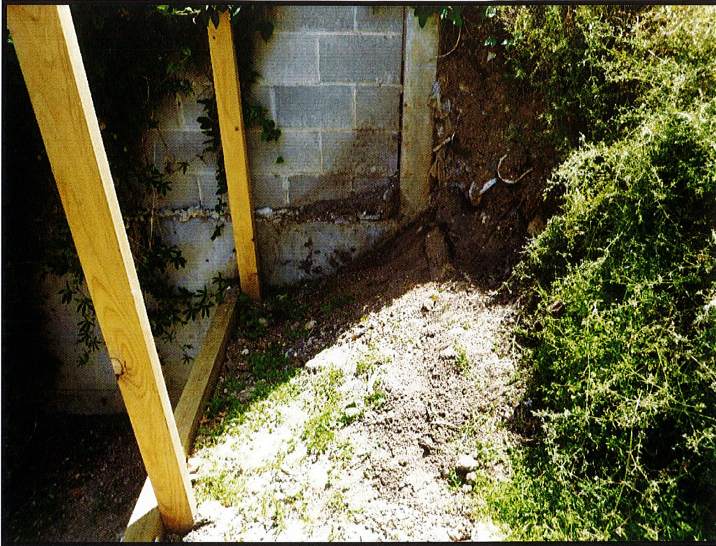
Photograph 9 – Photograph captured 19 November 2020. View of the western end of the subject land, looking west, at the north-east corner of 1 Campbell Grove (north-east corner of 1A Campbell Grove). Note vertical face of earth adjacent to concrete retaining wall.
