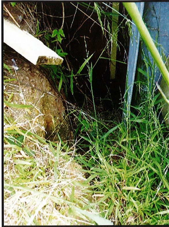
Photograph 21 – Photograph captured 13 October 2021. View of localised void beneath the south-east corner of the property boundary to 42 James Street, with the void appearing to extend beneath the south-west corner of property to the east of 42 James Street.
