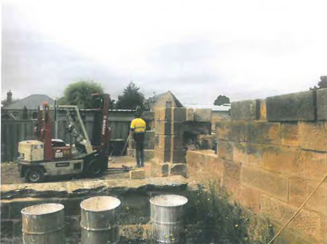
Commencement of the rebuild of the arch in its original location June 2013
